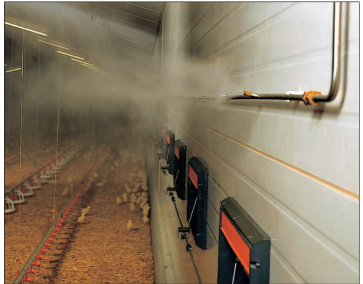
Using the Fogging Cooler system in a broiler house
